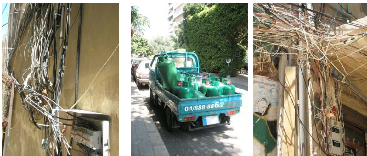
Pictures taken by the author of electricity wiring in Palestinian camps and gas distribution in Lebanon (middle)
